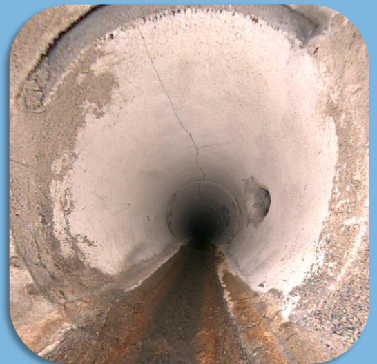
Top: CML lined pipe and laterals with cracking visible in concrete
